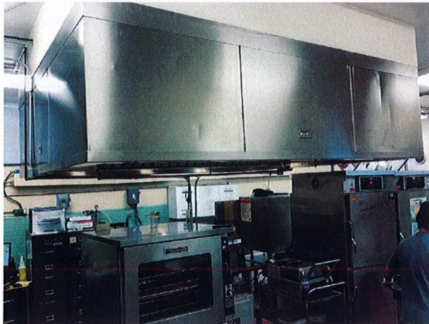
Pinnacle Figure 10: Kitchen hood
