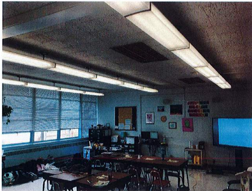
Pine Hall Figure 10: Surface mounted lights and no fire alarm devices
