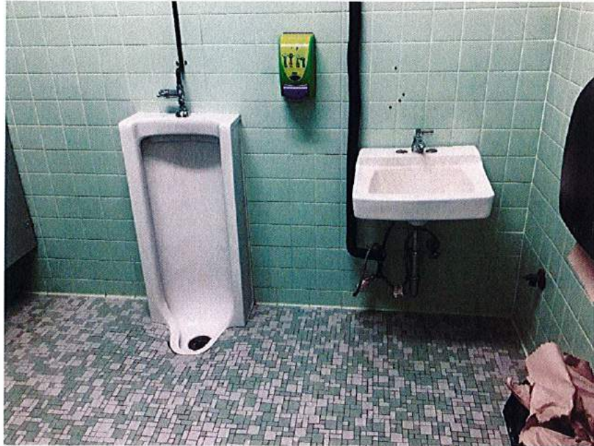
Pinnacle Figure 3: Exposed piping
