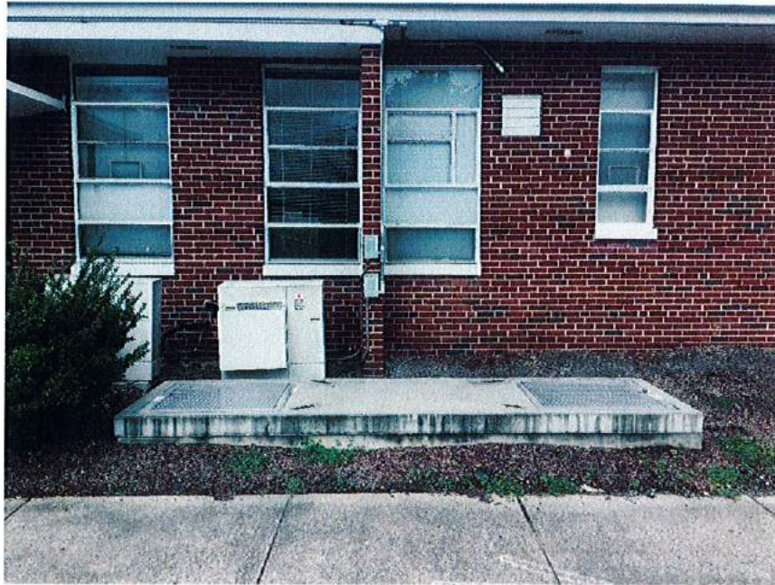
Pine Hall Figure 3: Grease trap and condensing units
