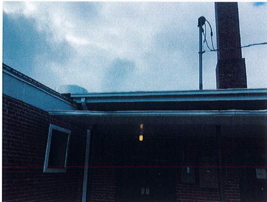
Pine Hall Figure 8: Main electrical service
