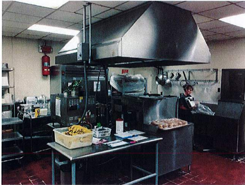
Lawsonville Figure 4: Tiny hood - No makeup air
