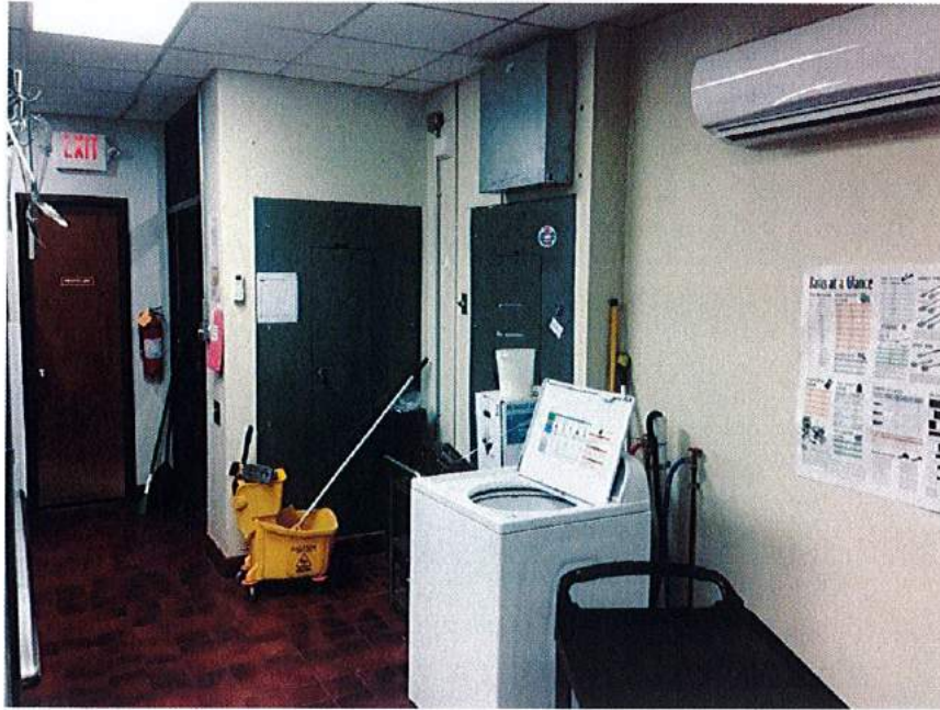
Lawsonville Figure 5: FPE Electric Panels
