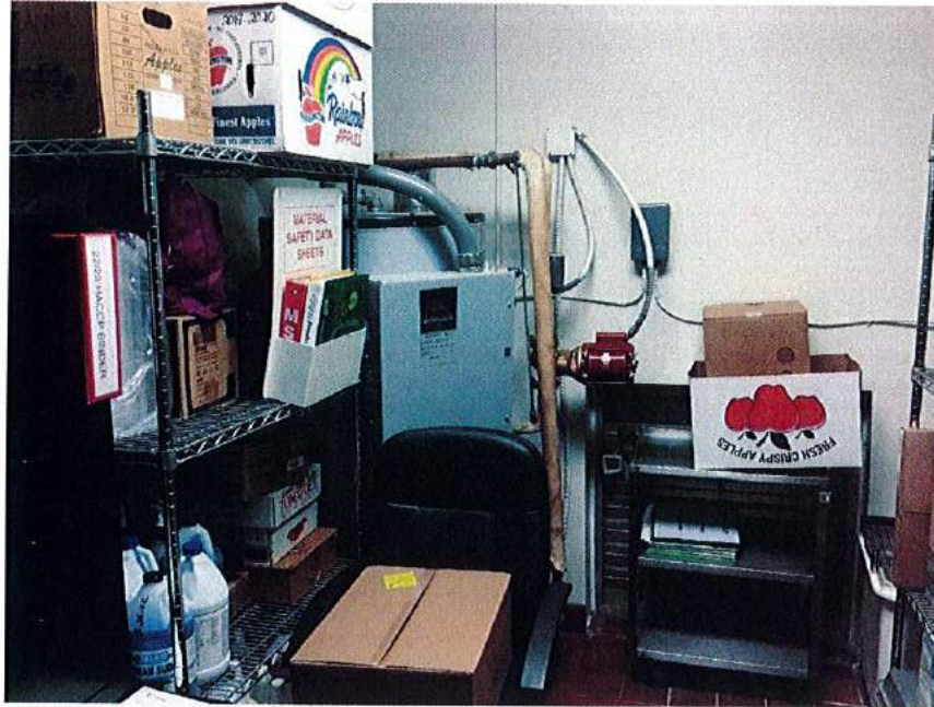
Lawsonville Figure 1: Electric Water Heater
